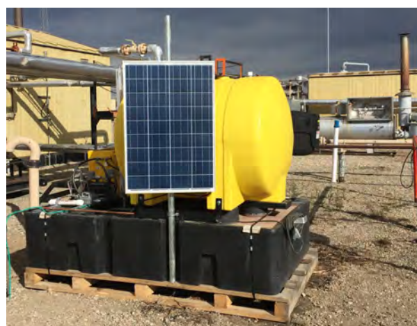
Figure 3: Solar chemical pump installed north of the 49th parallel
